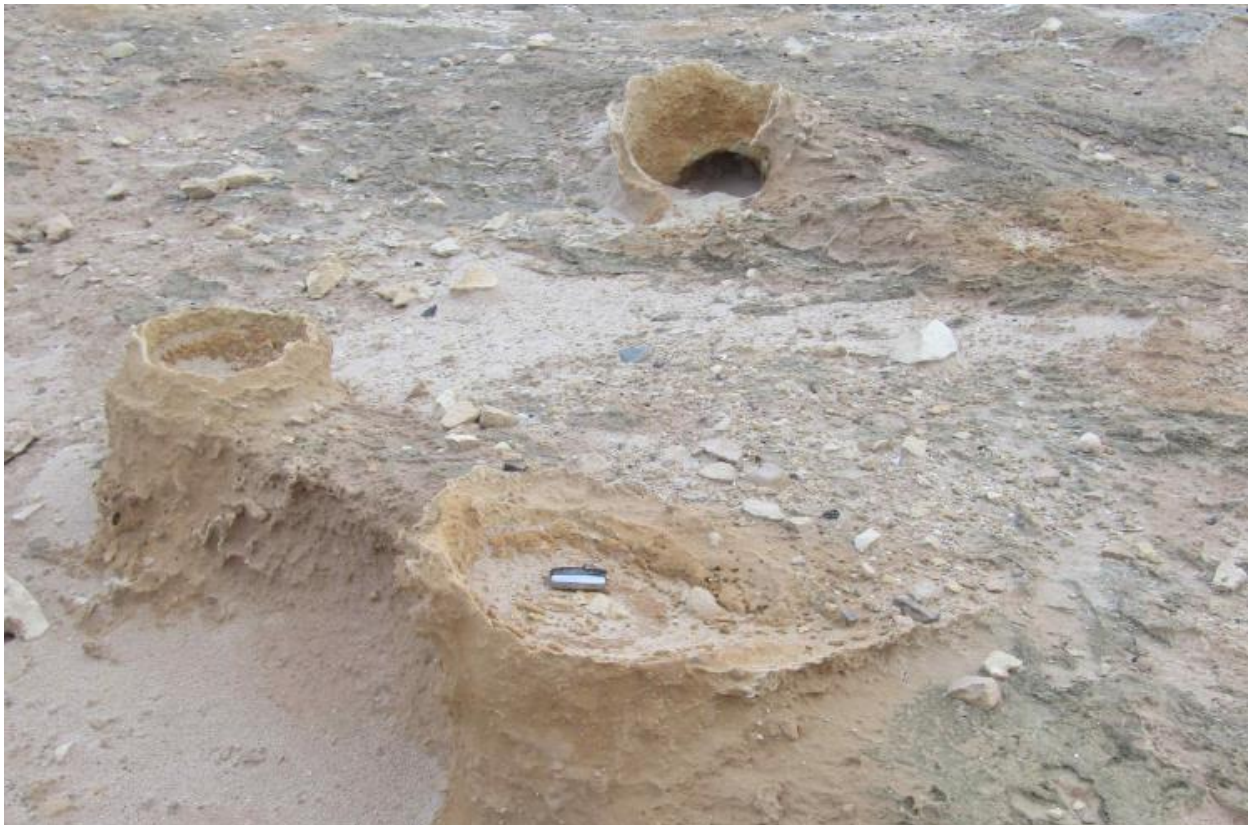
Figure 2. Top and bottom – the tops of the pipes protrude the calcrete layer (on Arniston East Shore).
