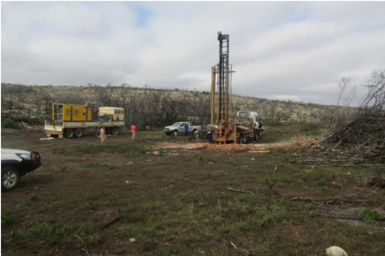
Figure 11. Drilling operations in the southern ravine, Patryskraal Farm. View to the southwest.
