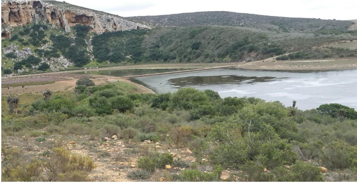
Figure 10. The concrete causeway. View to the southwest from the Riverbend Hill. (It was built during the 1950s next to the old, rocks causeway; Figure 11).
