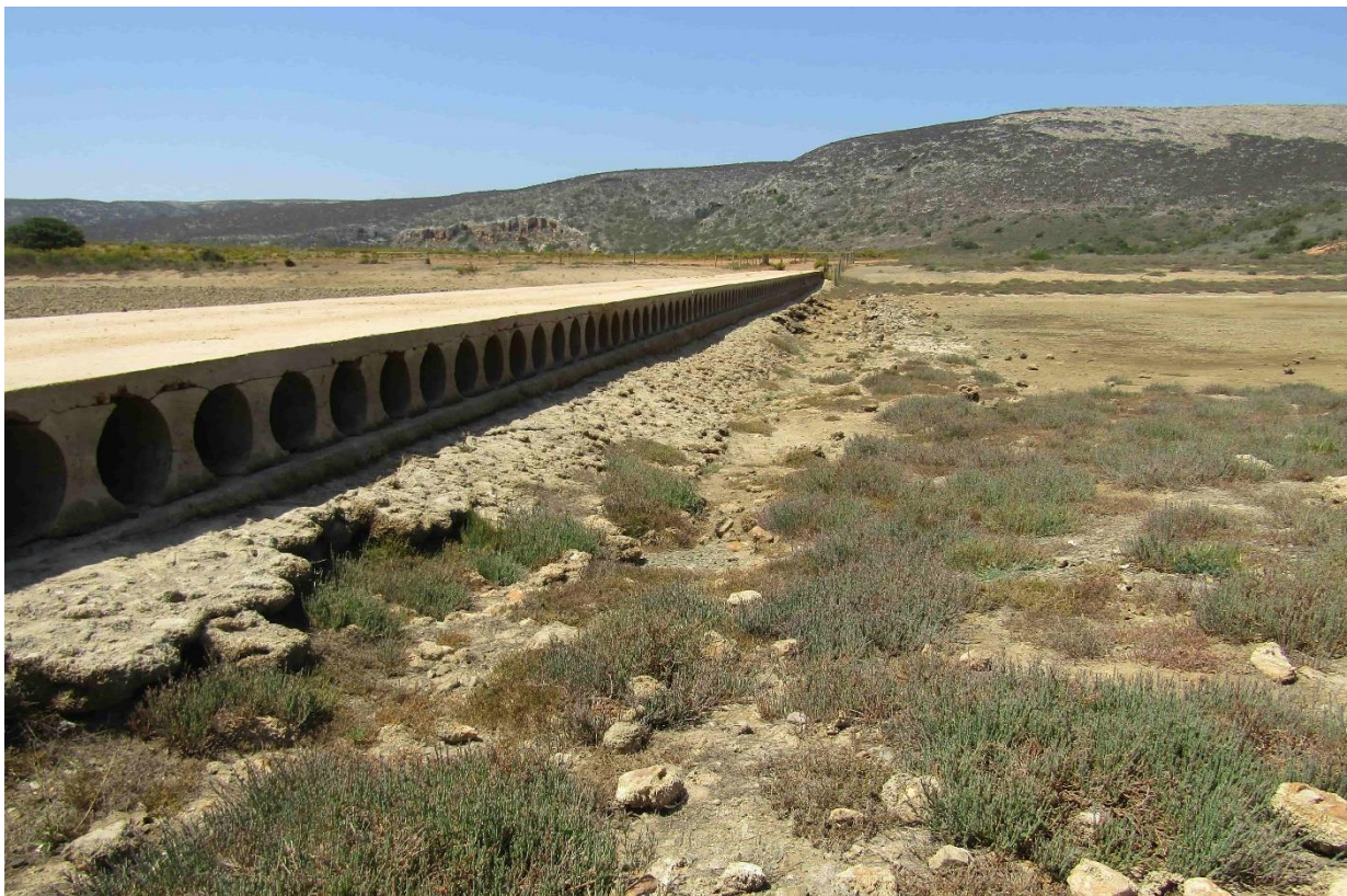
Figure 11. The concrete causeway is about 85 m long. View to the south. The old, rocks causeway can be seen to the right (west) side of the new one. The riverbed is ~9 m above sealevel and the top of the causeway is ~2 m above the riverbed, or ~11 m above sealevel.
