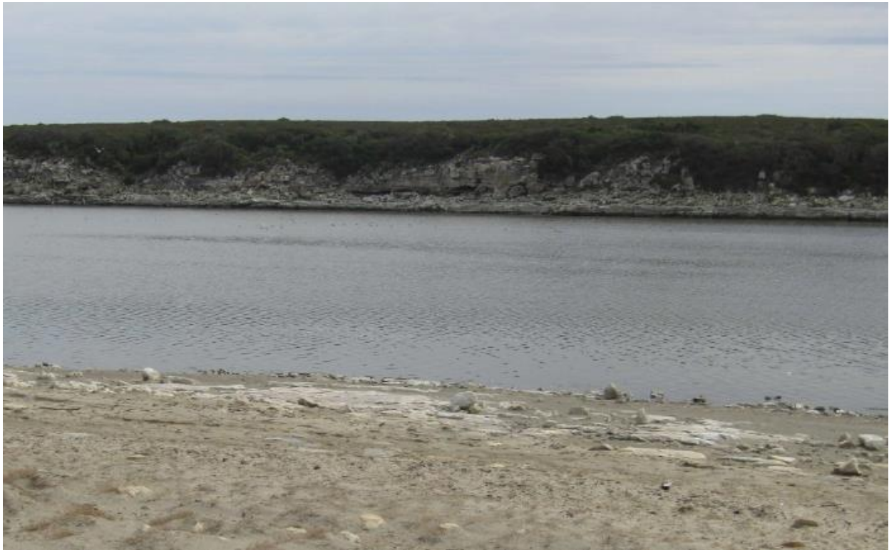
Figure 17. Nearly vertical wall on the east side of the southern section of the gorge.
