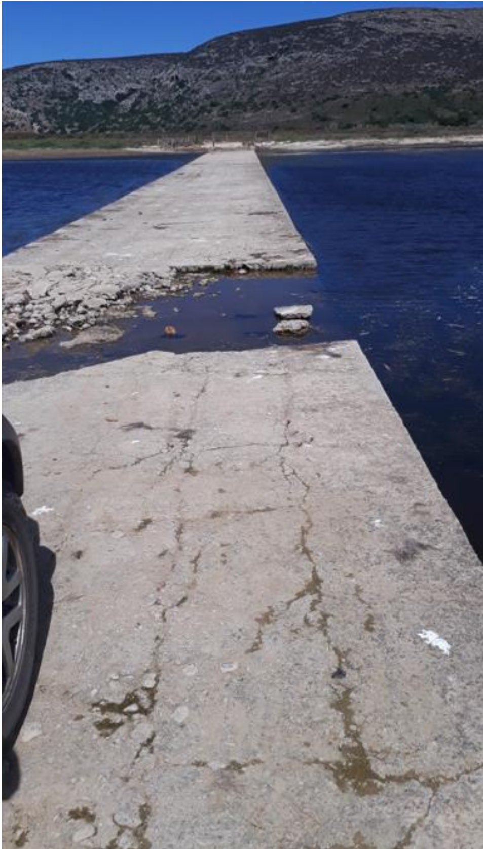
Figure 6. The damaged causeway.
