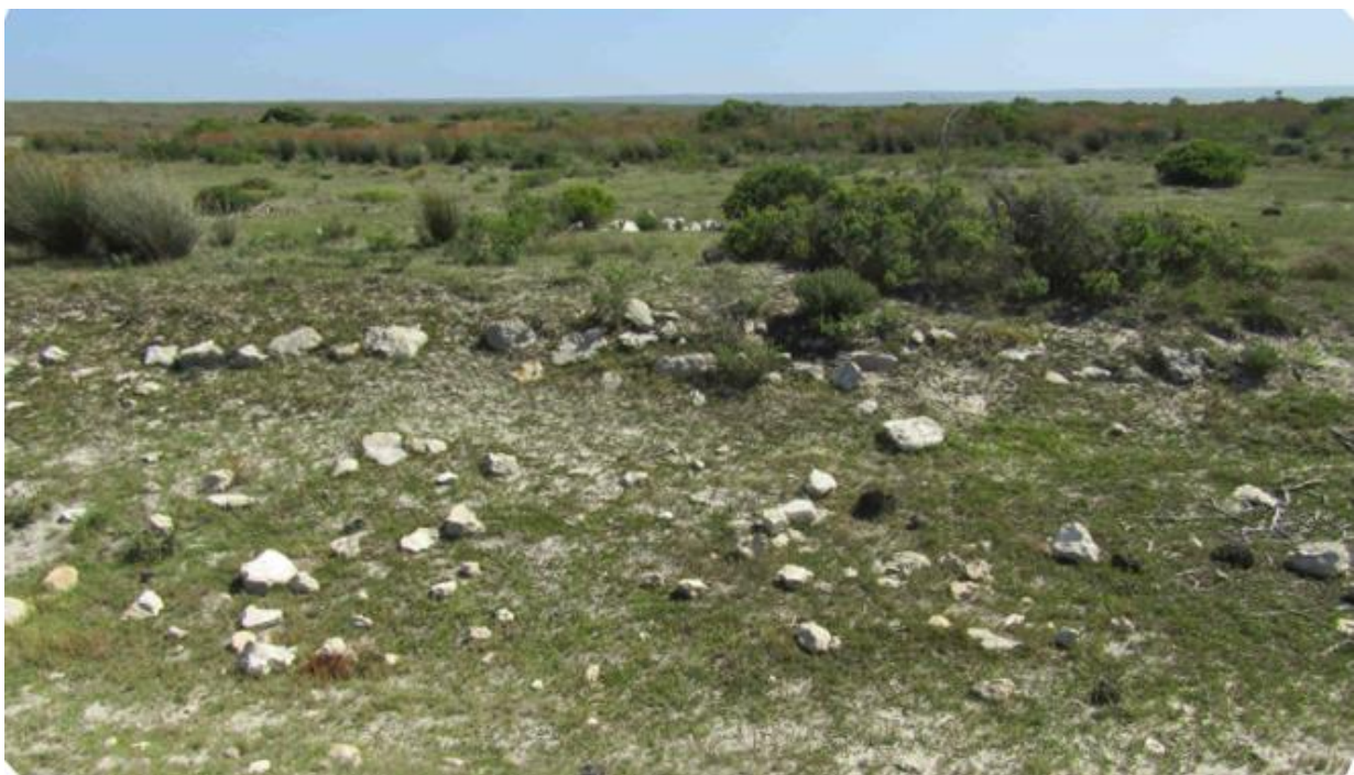
Figure 10. The walls of the canal were cladded with stones, to prevent erosion. The cladding disintegrated with time.
